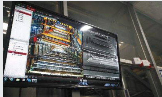
Infrared thermal imaging cameras and current monitoring system
