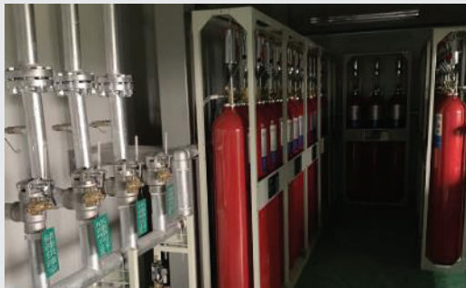
Fire warning and automatic fire extinguishing devices
